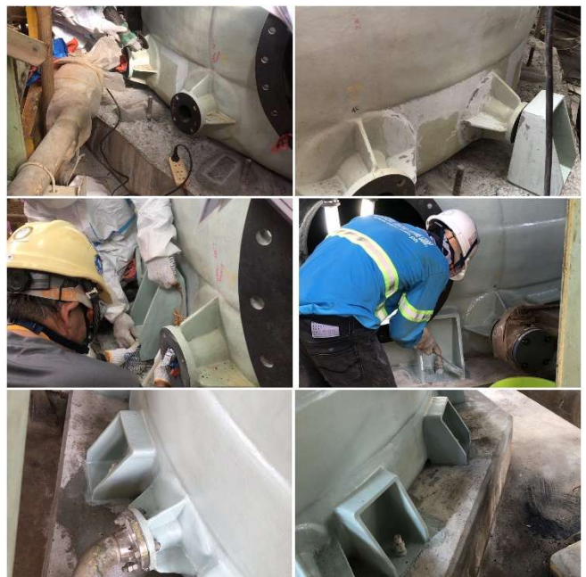
H2S Scrubber Tank Lug Lamination
