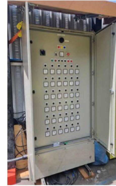
ELECTRICAL CONTROL PANEL
